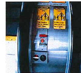
Know where to find emergency stop buttons.
